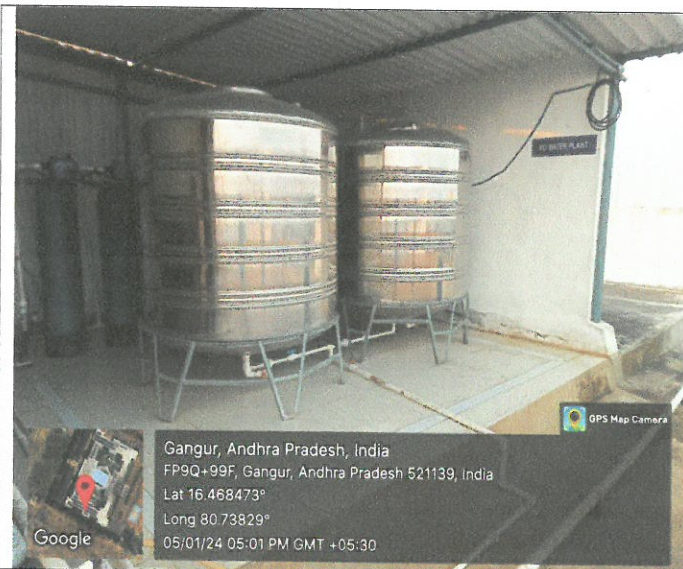
RO Water Plant
